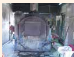
Quarantine incinerator - Port of Suva
