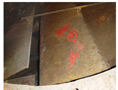
Photo 3. Fire damper unable to close.
