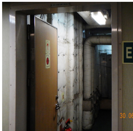
Photo 5. Fire door lashed open.
