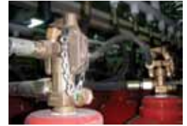
Transportation pins for CO 2 bottles of fixed fire fighting system not removed
