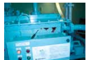
Sewage treatment plant tank walls corroded and holed
