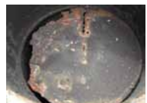
Defective fire damper
