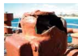
Damaged vent head
