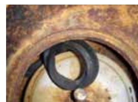
Water ballast tank air vent head rubber seat dislodged
