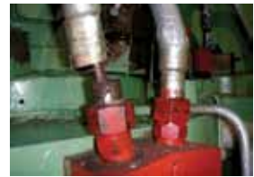
Damaged sheathing of main engine high pressure fuel oil pipe
