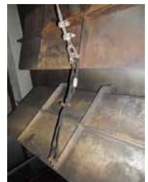
Funnel fire dampers closing arrangement defective
